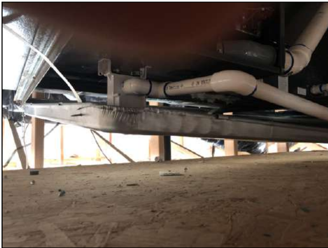
8.5 Item 5(Picture) No gas lines seen
