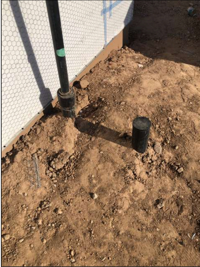
8.0 Item 1(Picture) Exterior clean outs
