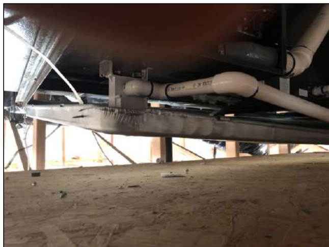
8.5 Item 5(Picture) No gas lines seen
